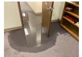
4. Water crept down the staff office hallway, and caused damage to Brad and Rosemary’s offices.
